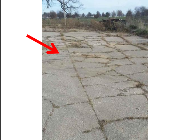
Photo 18: Further example of parking field conditions requiring replacement.
