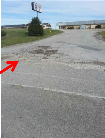
Photo 1: Example of deteriorating pavement surface at ingress/egress point.
