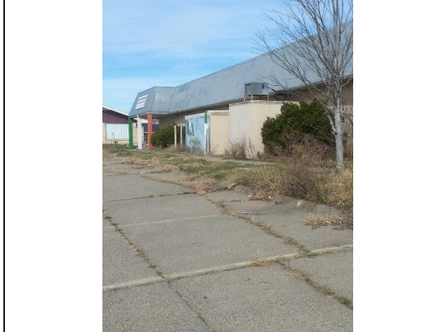
Photo 17: Further example of declining exterior conditions.
