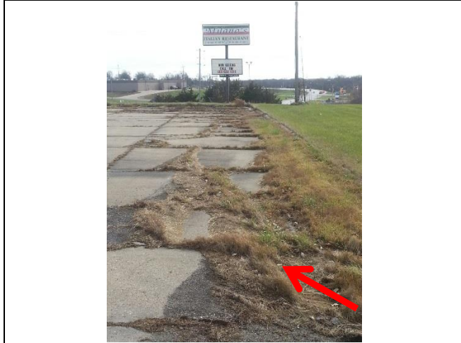
Photo 15: Parking field deterioration and cracking due to subsurface water penetration.
