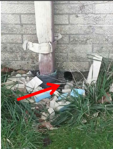
Photo 5: Example of debris and exterior hole providing access point for animals or rodents.
