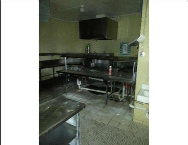
Photo 12: View of deteriorated and outdated interior conditions.
