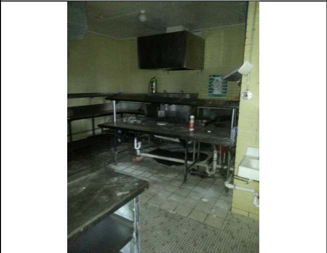
Photo 12: View of deteriorated and outdated interior conditions.
