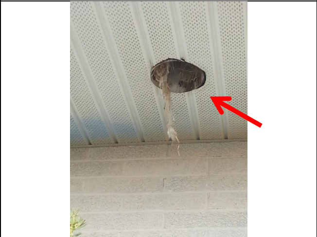
Photo 10: Additional example of electrical issues and where birds have access soffit
