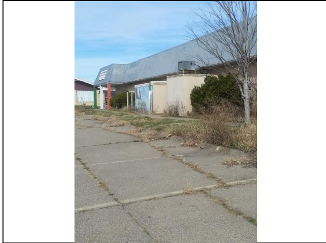
Photo 17: Further example of declining exterior conditions.
