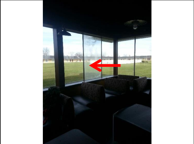
Photo 16: Example of window with broken seal.
